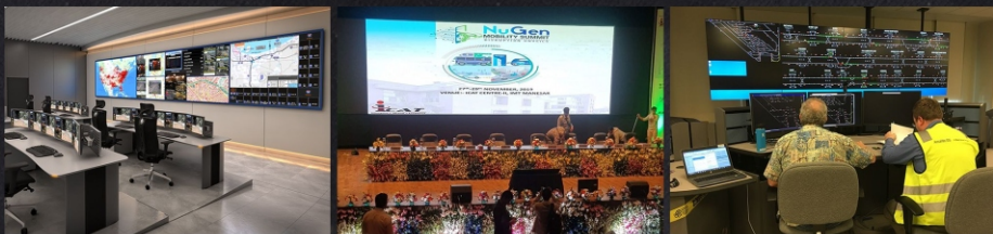
Command & Control Room
